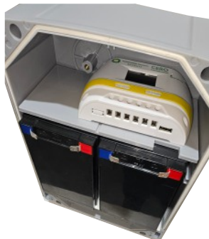
Plastic shelf on top of batteries with regulator placed on top
